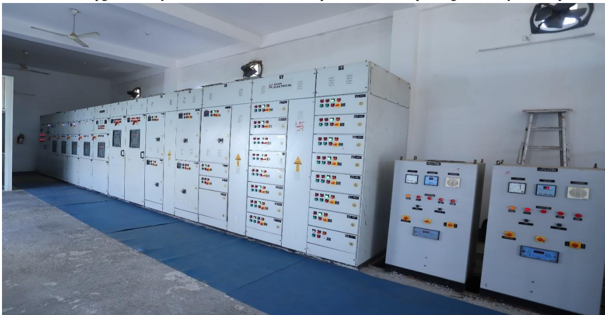
IPS Control Panels, Ghaziabad
